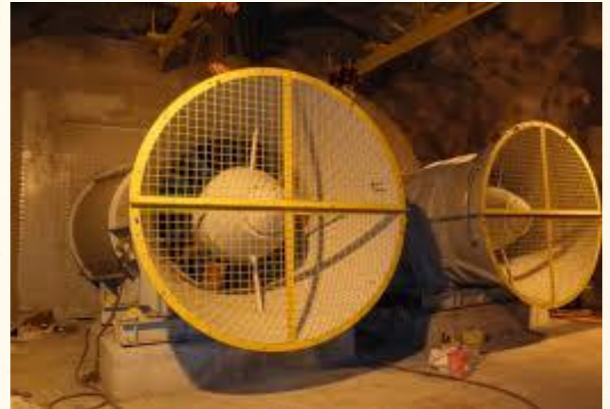
Main fans. Source: CPC Engineering
