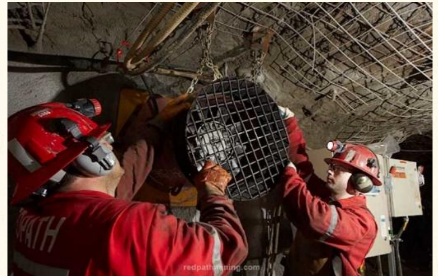
Auxiliary fan. Source: Redpath Mining
